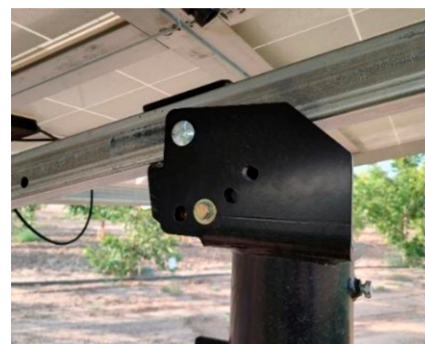
Fig. 2. Connecting hinge of steel racking system that allows manual adjustment of tilt installed photovoltaic modules.
