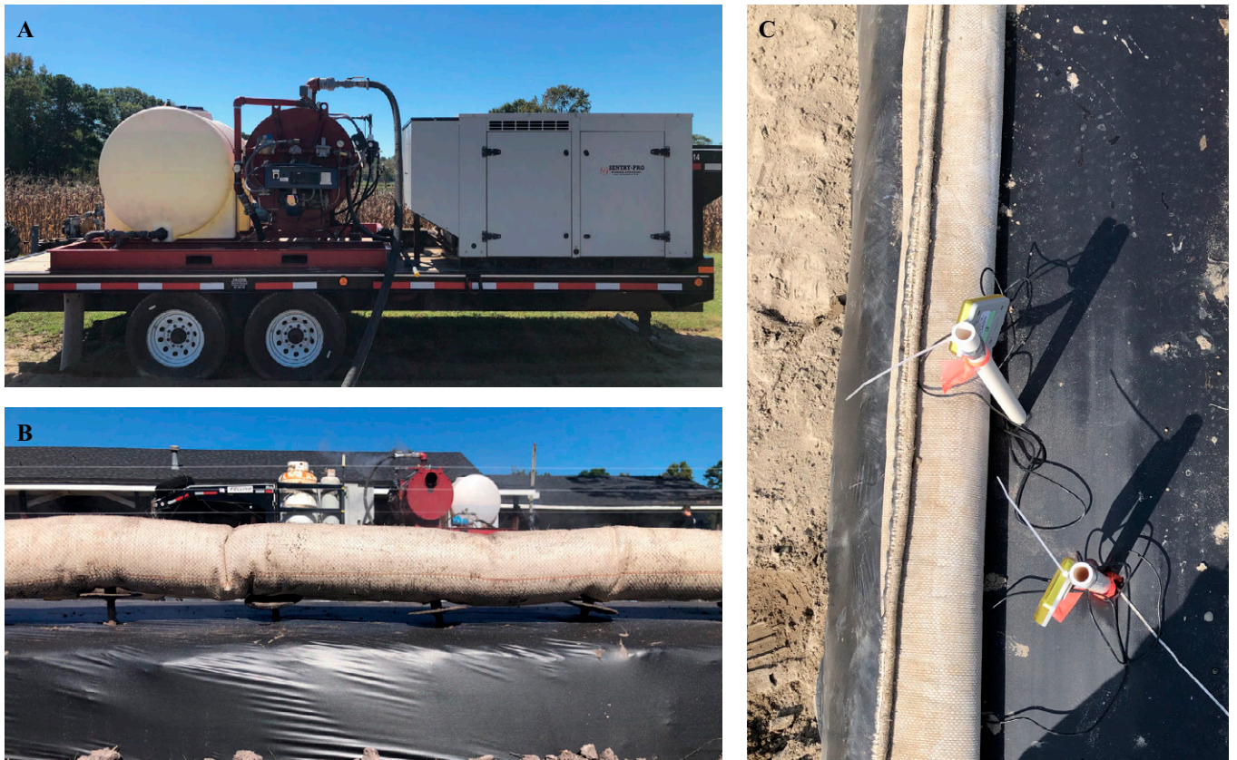
Fig. 1. Steam generator and field application. (A) Sioux® Steam-Flo 25L Boiler (Beresford, SD, USA). (B) Spikes injecting steam into a raised bed. (C) Spike hose applied on both sides of the raised plastic bed.
