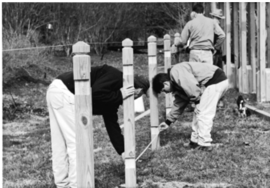
Fig. 1. Students work in teams of four to five students, often solving problems during actual construction.
